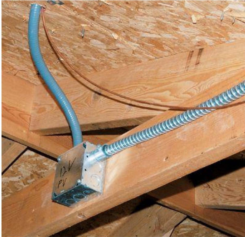
The feed wires from the collector are fed into a junction box inside the structure where connections to the power distribution equipment are made.
