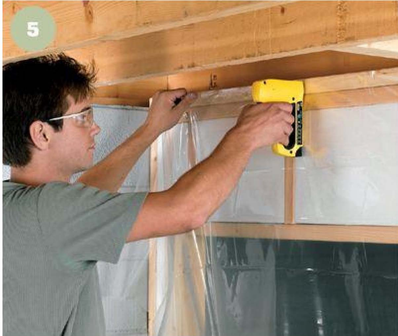
5 Staple a sheet-plastic vapor barrier to the basement side of the walls where condensation is likely to form.
