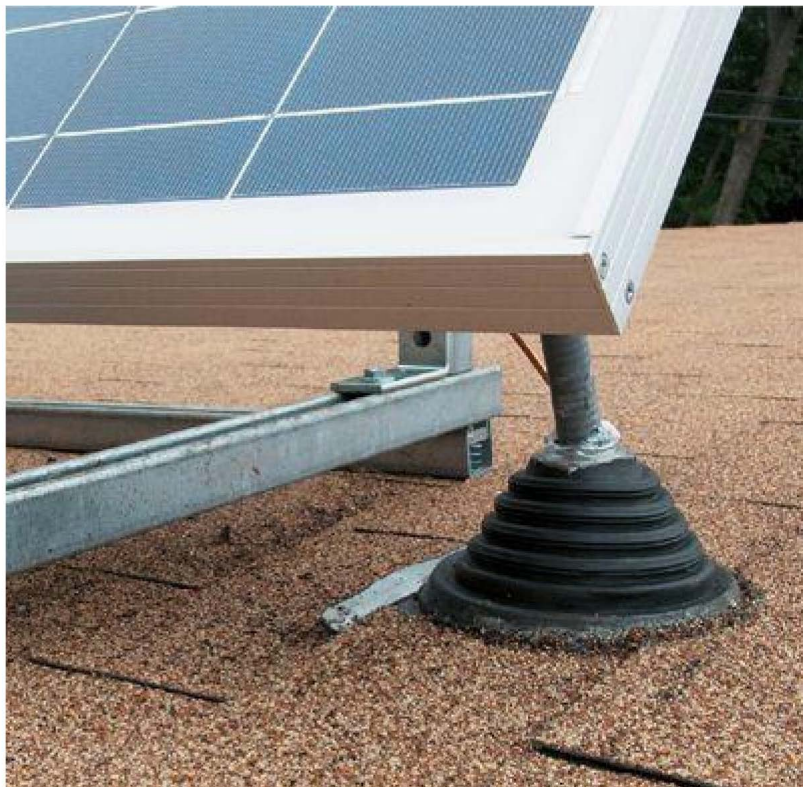
An EPDM rubber boot seals off the opening where the PVC conduit carrying the feed wires penetrates the roof.
